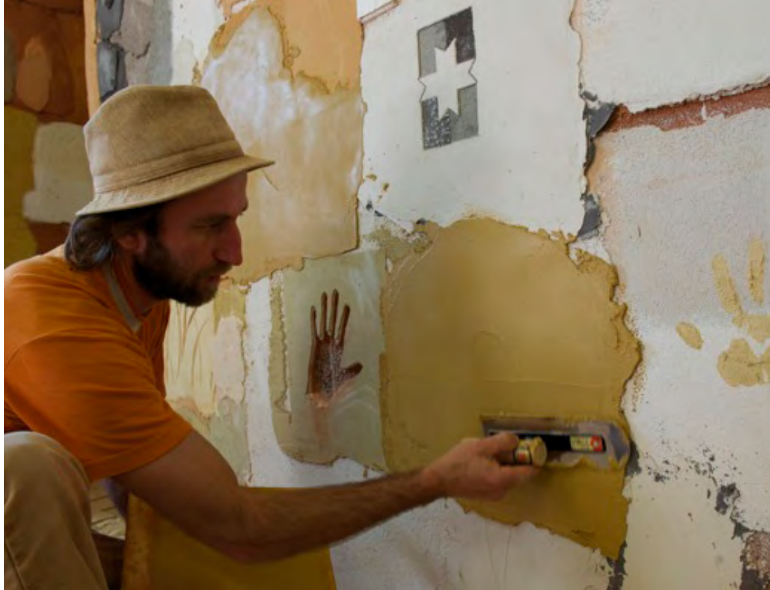
Masterful clay plasterer Marko Kikas applying his skills on a wall in Mooste. Põlvamaa
